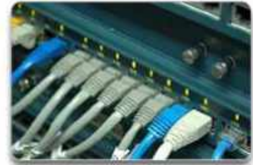
Cables must be connected correctly.
